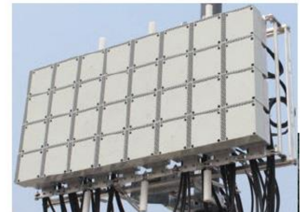
Massive MIMO antenna array for a Huawei 5G field trial.
